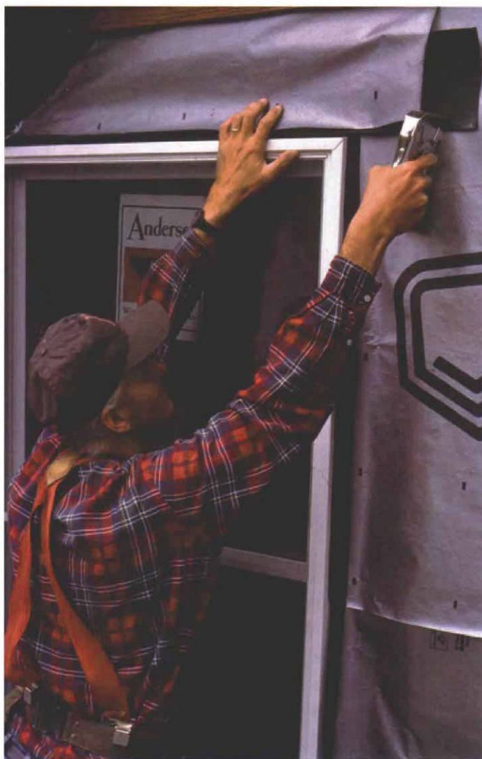
Yes, some windows can be flashed with tarpaper and housewrap. Lapping asphalt-felt paper and housewrap over the nailing flange of this clad window will help keep water out of the framing.
